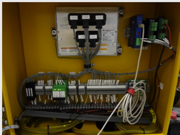
E3 control system installed on the G3408.
