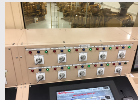
Fig. 2.2 Engine Control Panel
