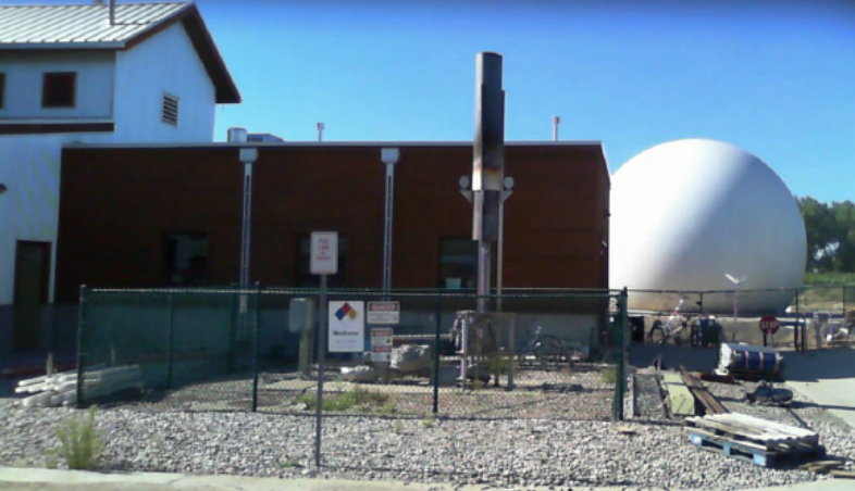
Single digester & flare at water treatment facility.
